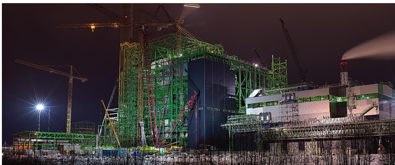
A LARGE PROJECT IN PROGRESS, DUE TO BE COMPLETED IN 2014: CONSTRUCTION OF POWER SYSTEMS WITH NECESSARY EQUIPMENT FOR OIL SHALE AND BIOFUEL HANDLING SYSTEMS IN THE TERRITORY OF ESTONIAN POWER PLANT.
