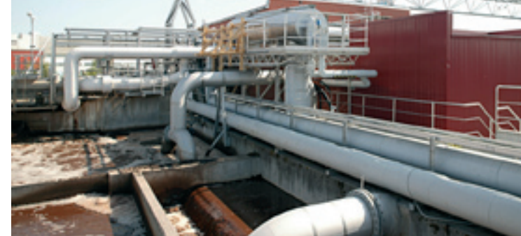
YIT supplied water treatment equipment for a thermal power plant in Myllykoski on behalf of Vamy Oy.
