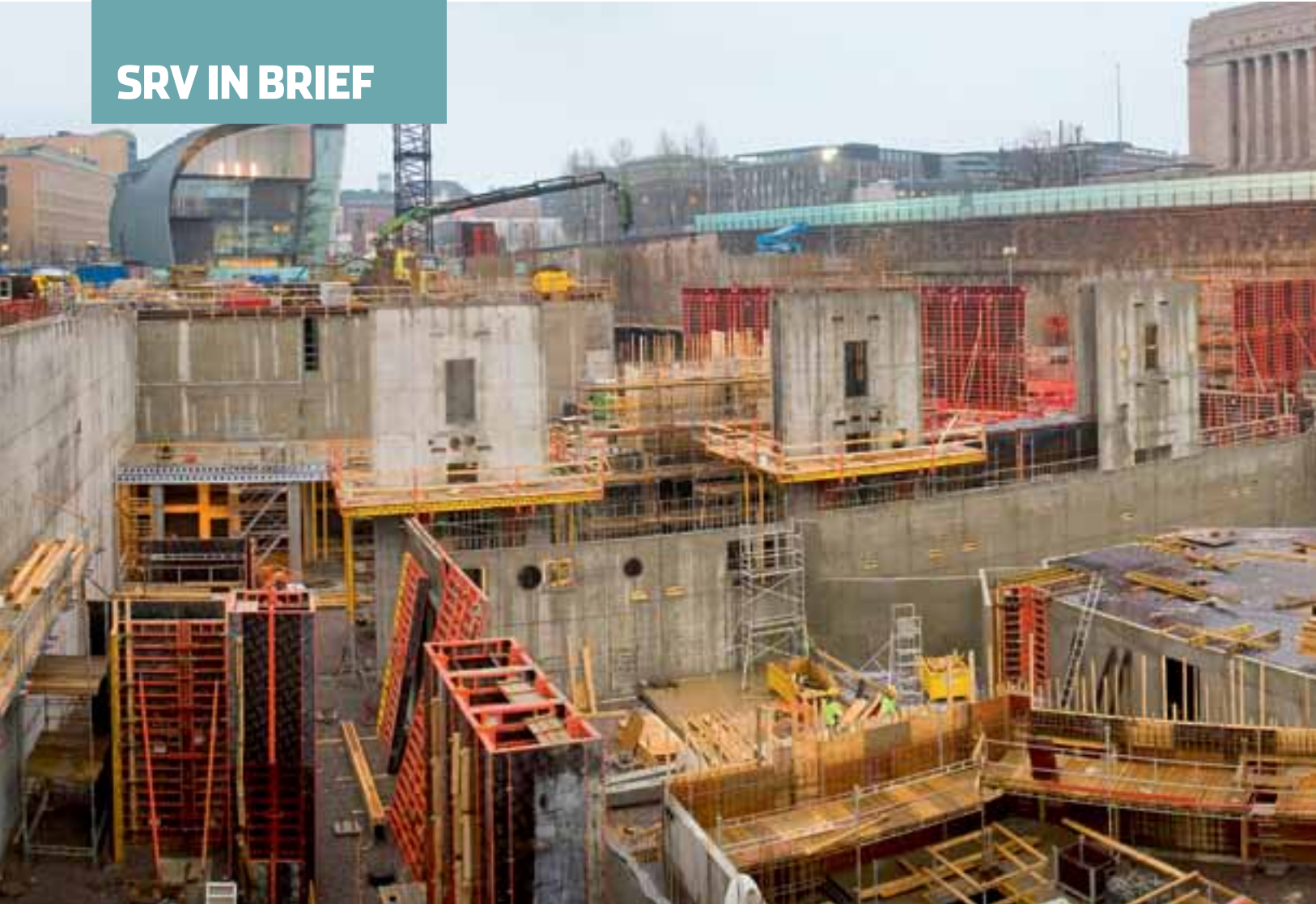
The construction of the Music Centre was started up in the centre of Helsinki in the autumn.
