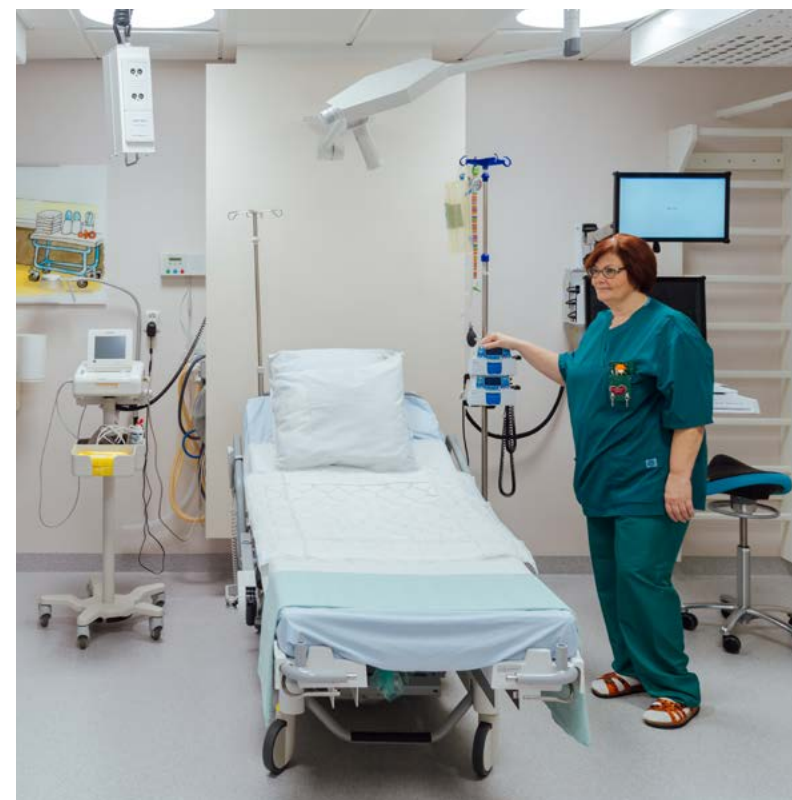
In the modernised delivery rooms, all the equipment required is within reach of the midwives.
