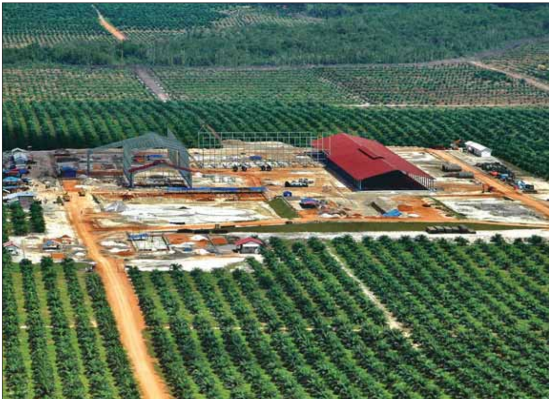
An aerial view of the Palm Oil Mill under construction in PT SSSI, Indonesia.
