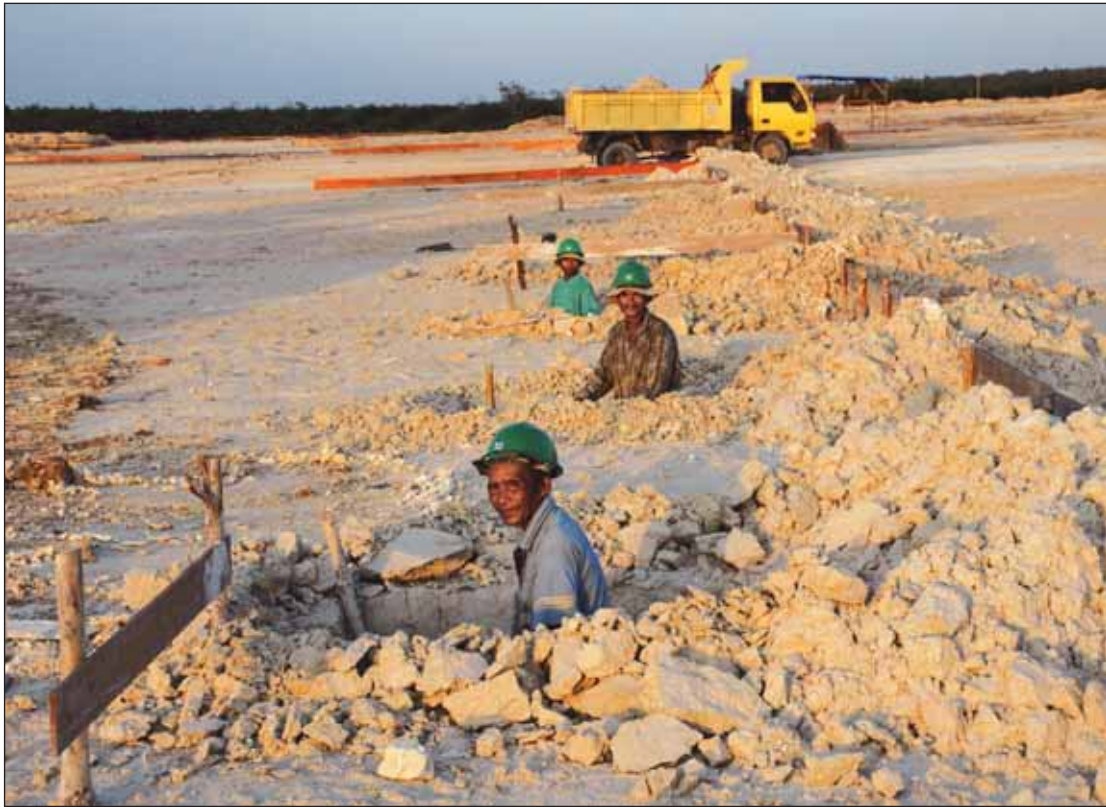
Foundation pits for the new Palm Oil Mill's steriliser station being dug out manually in PT SSSI, Indonesia.
