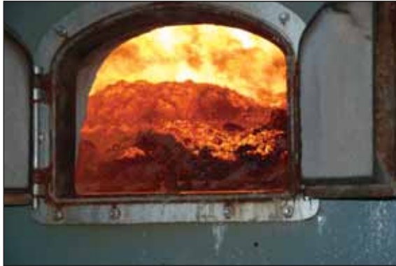
Fibre, Shells and Empty Fruit Bunches being converted into Green Electricity.
