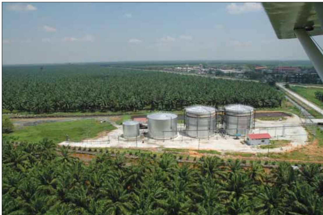
A Biogas Plant at Jendarata Estate treating the Palm Oil Mill Effluent. In the process of reducing the Biochemical Oxygen Demand by 99%, biogas is produced by methane bacteria and subsequently used as a source of green energy.
