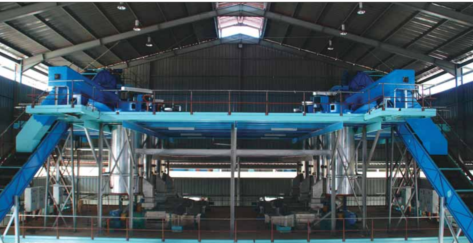
PT Surya Sawit Sejati's "State of the Art" Palm Oil Mill under construction in Lada, Central Kalimantan, Indonesia.
