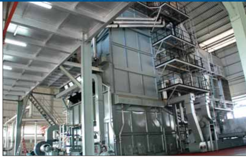
The well laid out Biomass Boiler at Jenderata Estate.
