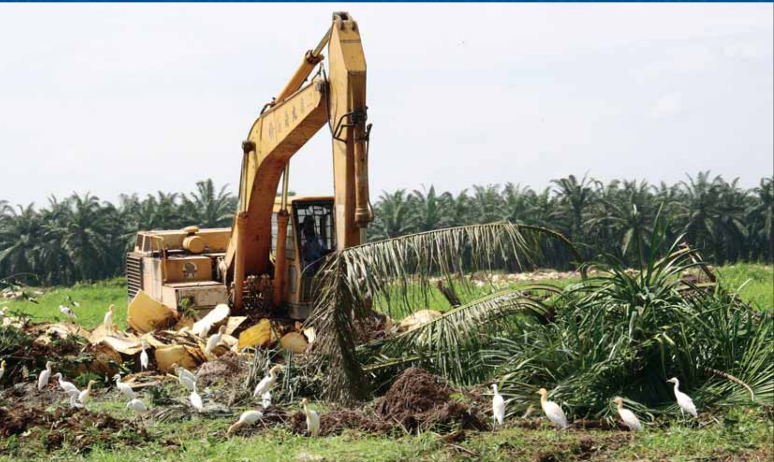
A hydraulic excavator chipping the trunks of the old stand in support of our zero-burn policy. The chips are recycled as mulch which adds organic matter and retains moisture.
