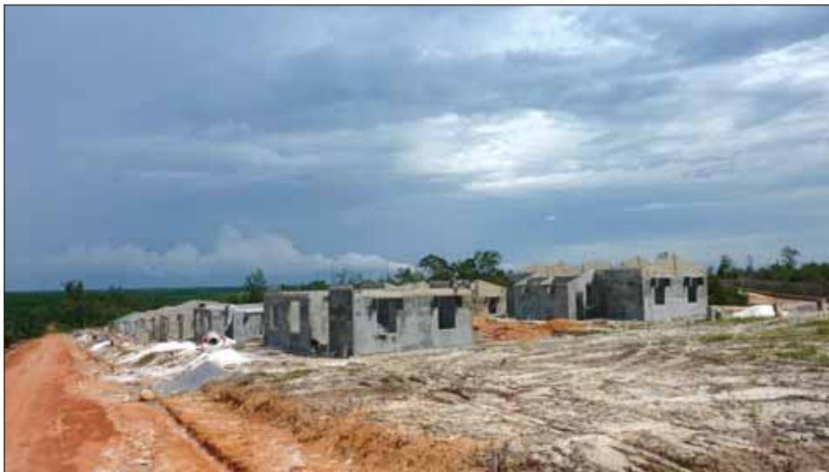
First phase of semi-detached concrete workers' houses in progress at Lada Estate, Indonesia.
