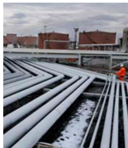
The production plant at Mongstad is an important hub for the refining and export of Norwegian crude oil.
