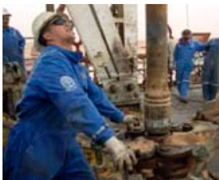
The first drilling location in Hassi Mouina HTJ-2, Algeria in 2006. We are operator for the exploration phase in the Hassi Mouina licence.
