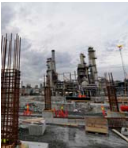
StatoilHydro, Gassnova, Dong Energy, Shell and Vattenfal have signed an agreement to build a full-scale carbon capture plant at our refinery at Mongstad.
