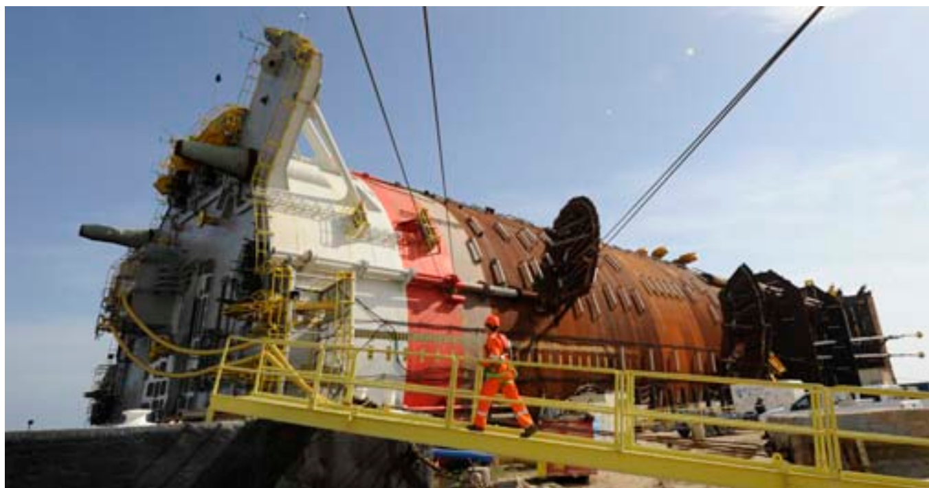
At the yard in Corpus Christie, work is underway to complete the Tahiti platform for production start in the Gulf of Mexico in 2009.
