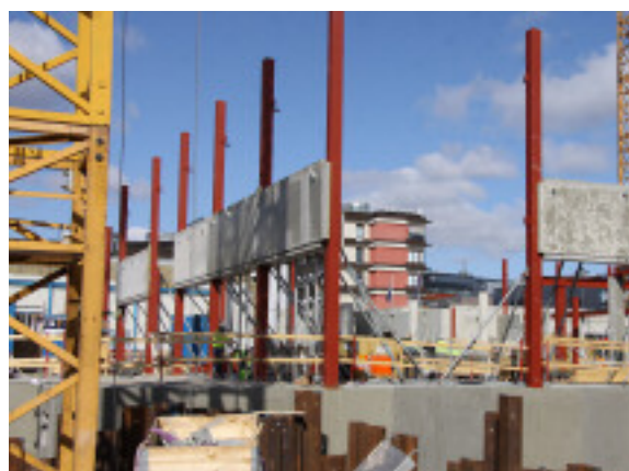
Kista Isafjord 1: Ongoing new construction and refurbishment of a new office building for Ericsson totalling 36,000 sq.m. Occupation is estimated at April 2012.
