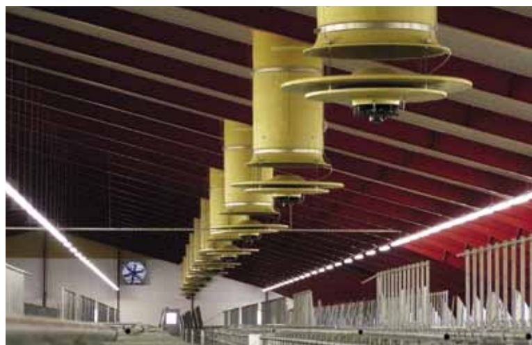
Air Inlet / Recirculation Chimney
