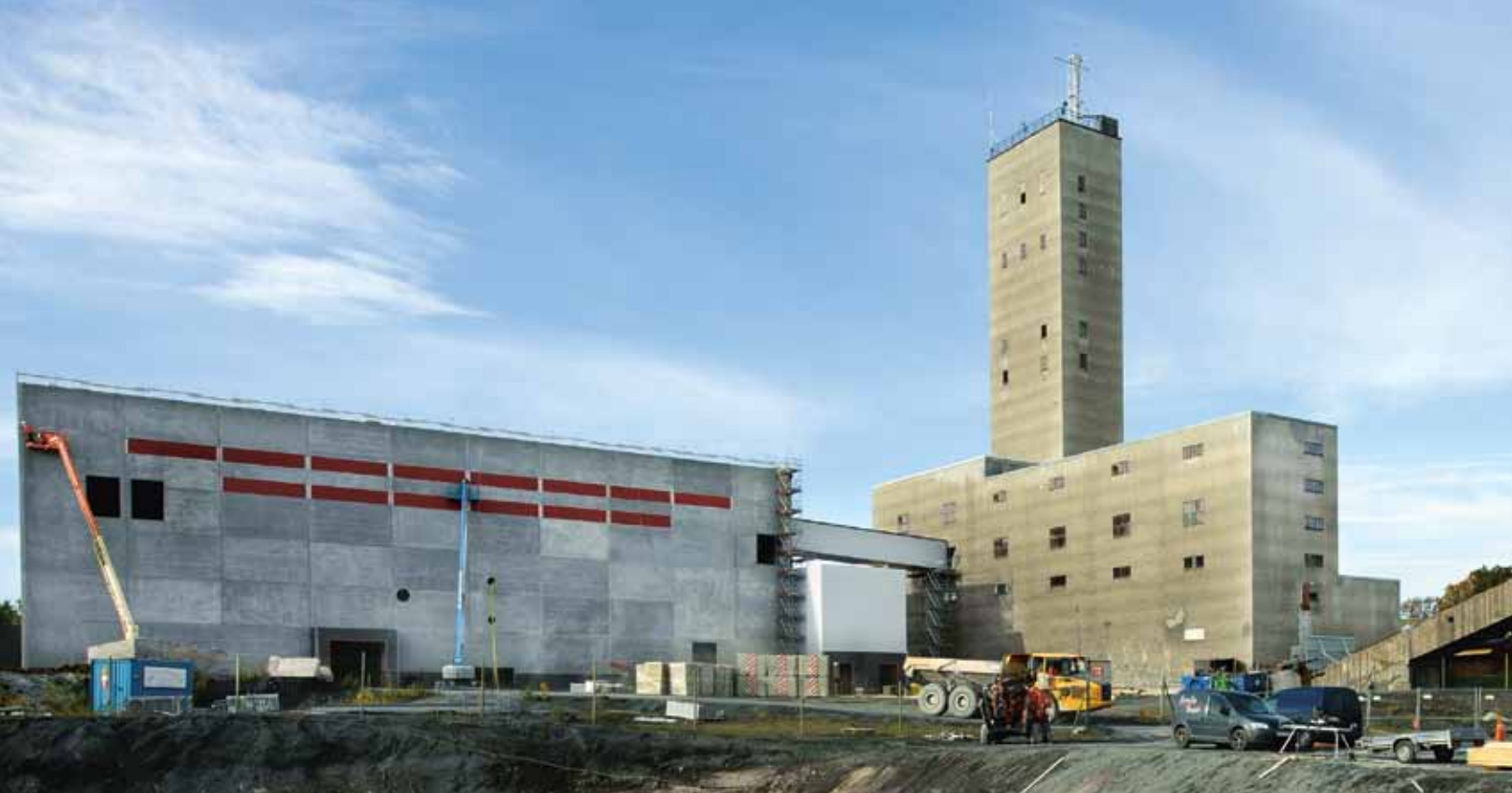
Trial operation and running-in at the new sorting plant started in March 2012.
