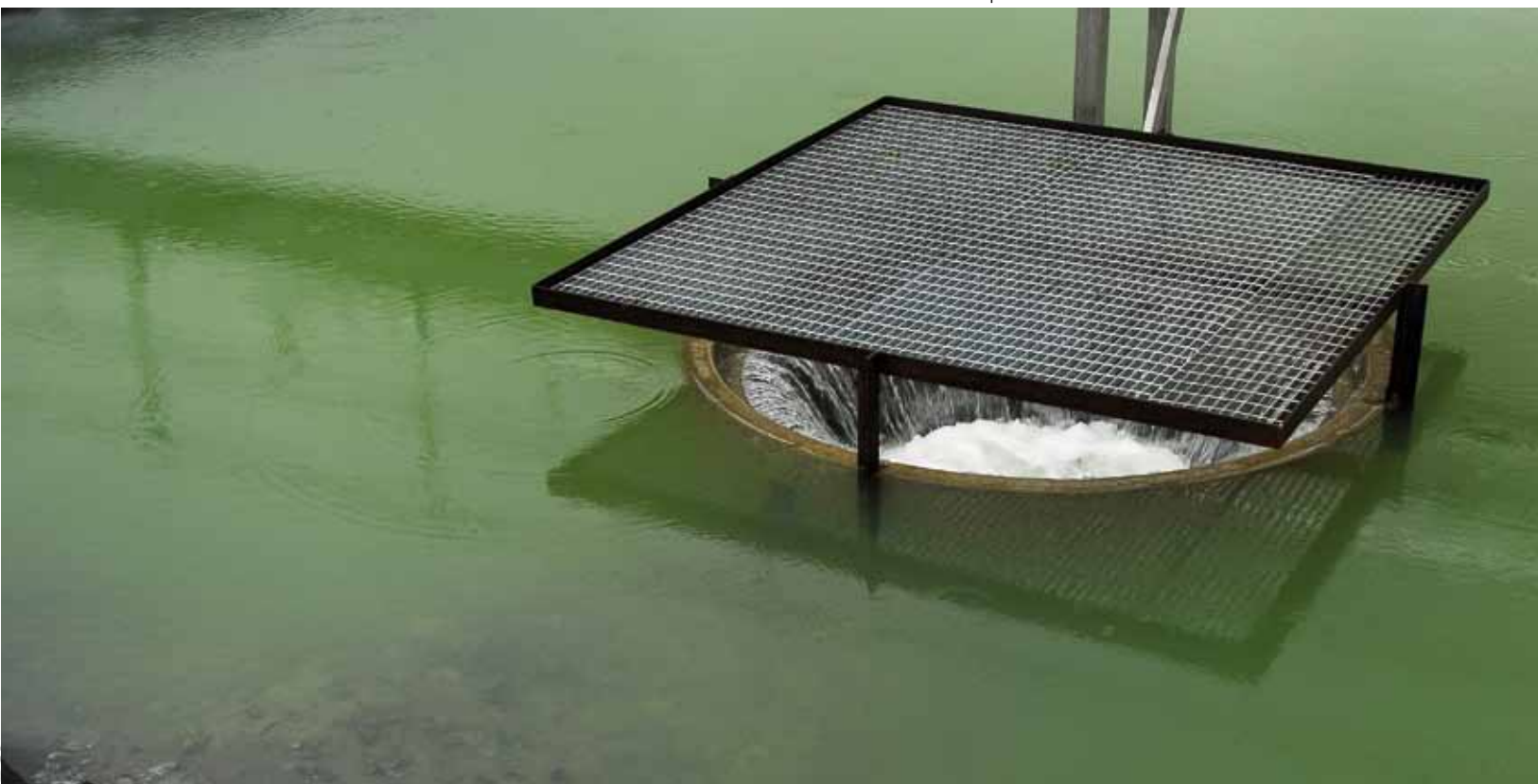
Outflow of the purified water from the sedimentation basin.
