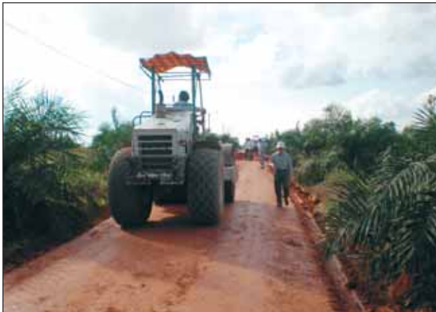
The Senior Executive Director, inspecting road construction works taking place in Lada.
