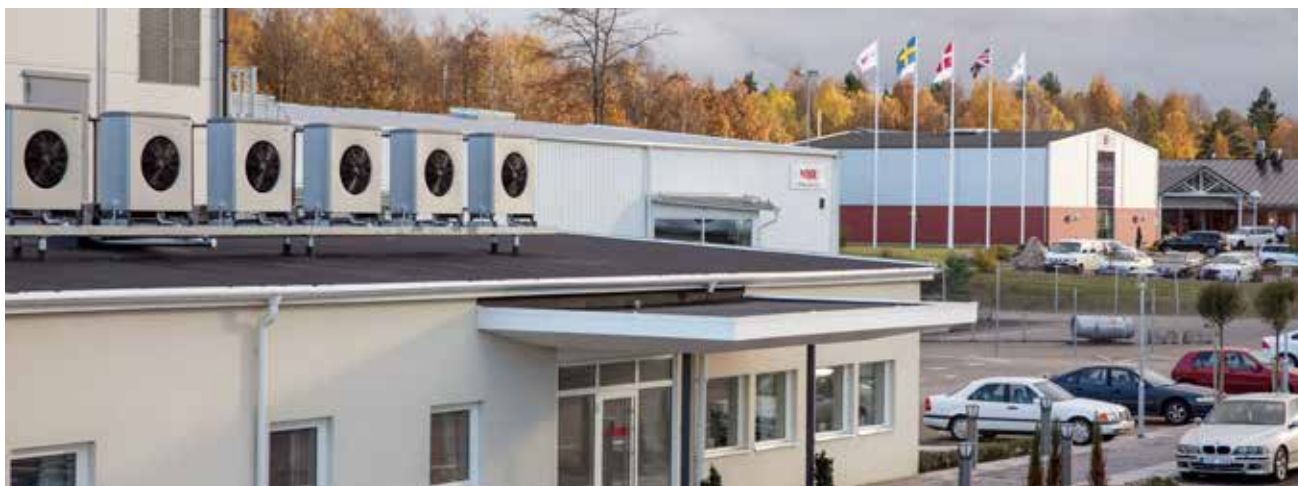
In 2012 a brand new heat-pump array was installed at the Heat-pump Plant in Markaryd. The array produces 180 kW of heat from energy taken partly from five 160-metre deep boreholes and partly from the outside air with the aid of six NIBE AMB air collectors of around 20 kW each. Energy is also recovered from the air used when function-testing products as part of the manufacturing process.
