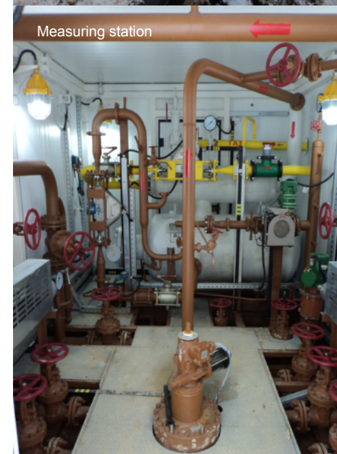
Shelton infield pipeline from well to facilities
