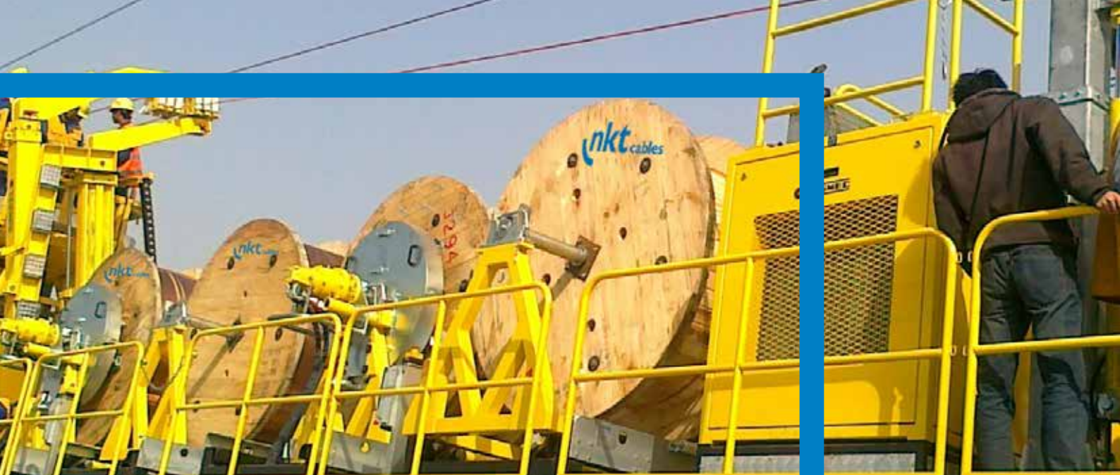
Installation of catenary wire on high-speed rail link between Shanghai and Beijing
