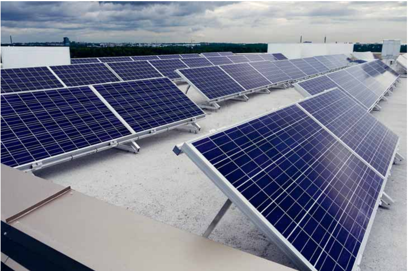
Kaukomarkkinat delivered a solar electricity system of more than 40kW to SRV's Derby Business Park in Espoo, Finland.
