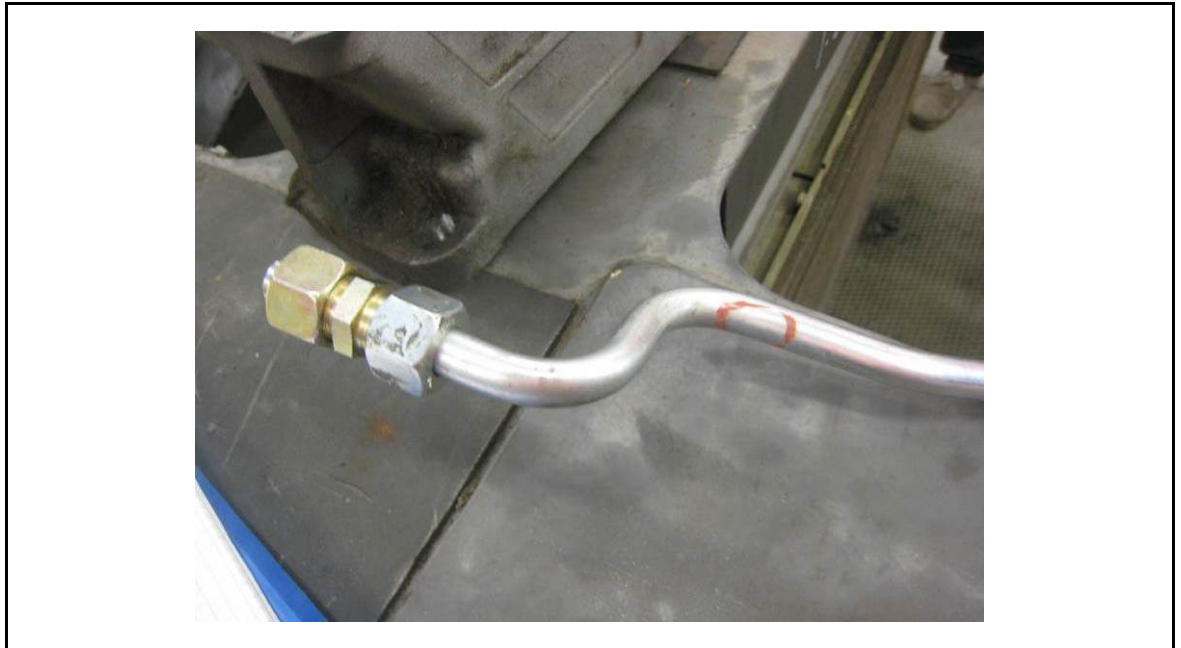
figure 10-15: Area in the fuel pipe where the leakage appears (PROSE)
