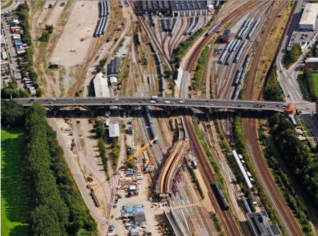
In the railway cutting west of Aarhus Central Station, Aarsleff constructs a 125-metre long bridge leading the city's future light rail transit across six railway tracks.
