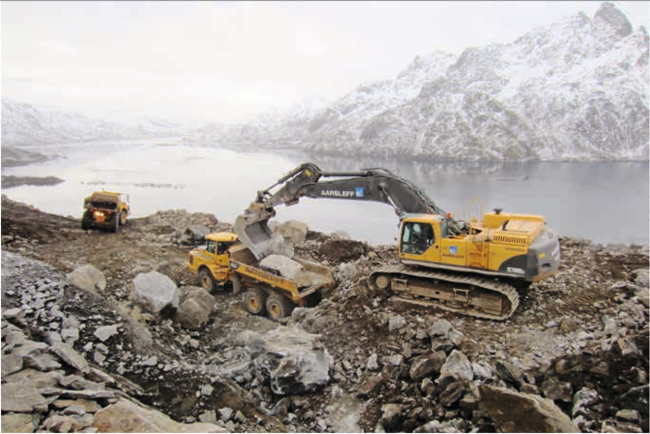
Aarsleff extends the fishing port in the village of Myre in Vesterålen in Norway and establishes new stone breakwaters.
