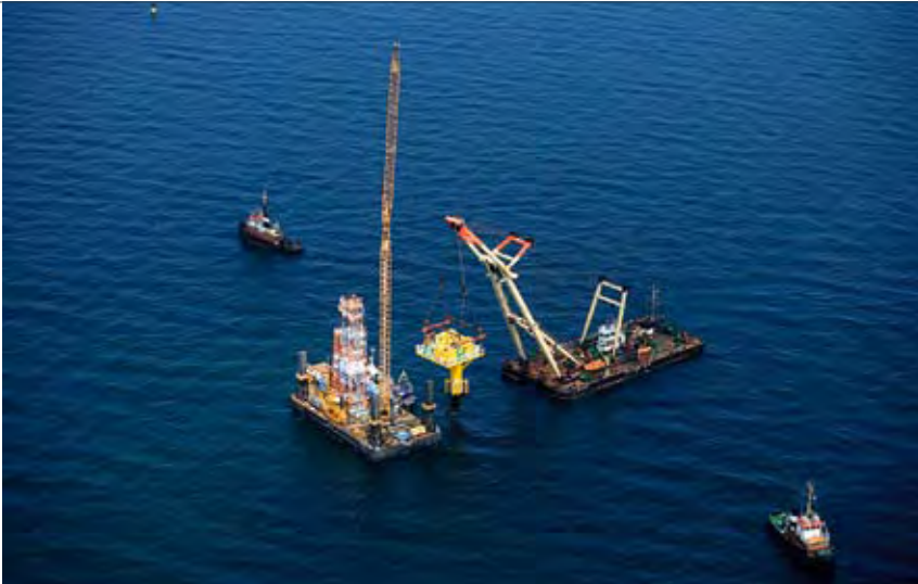
On Krigers Flak, in the waters between Bornholm and Rügen, the German research and anemometer mast Fino 2 was completed and handed over.
