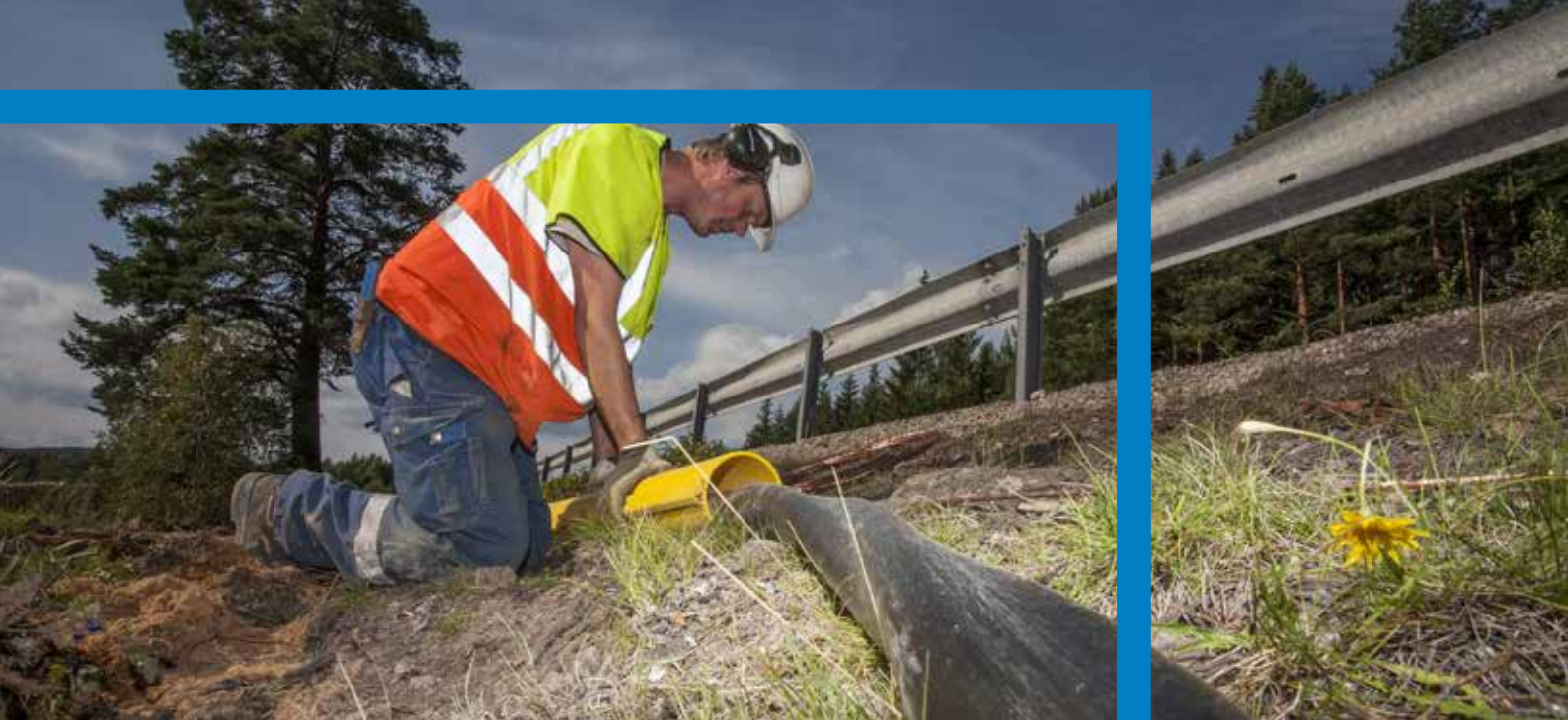
Extending and reinforcing the distribution network while constructing a new section of highway
