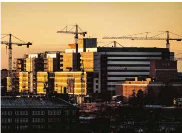
Controlling a huge hospital. The 330,000 square metres New Karolinska Solna hospital is currently one of Europe's largest buildings. Building service systems of the highest quality are required to manage the operation of a facility as important and complex as a large, modern hospital. Sweco has had the challenging task of preparing all systems to work together. Systems for heating, cooling, ventilation and much more will communicate with each other to ensure the safest and most efficient hospital operation possible.
