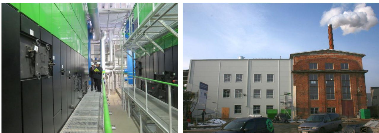
Photo: new biofuel boilers and renewed Inkaras boiler-house building
