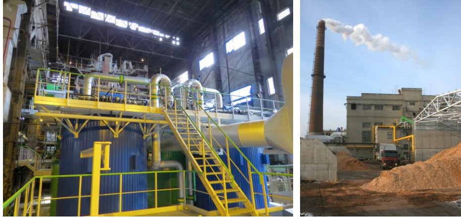
Photo: new water heating boilers and biofuel depot in Petrašiūnai power-plant
