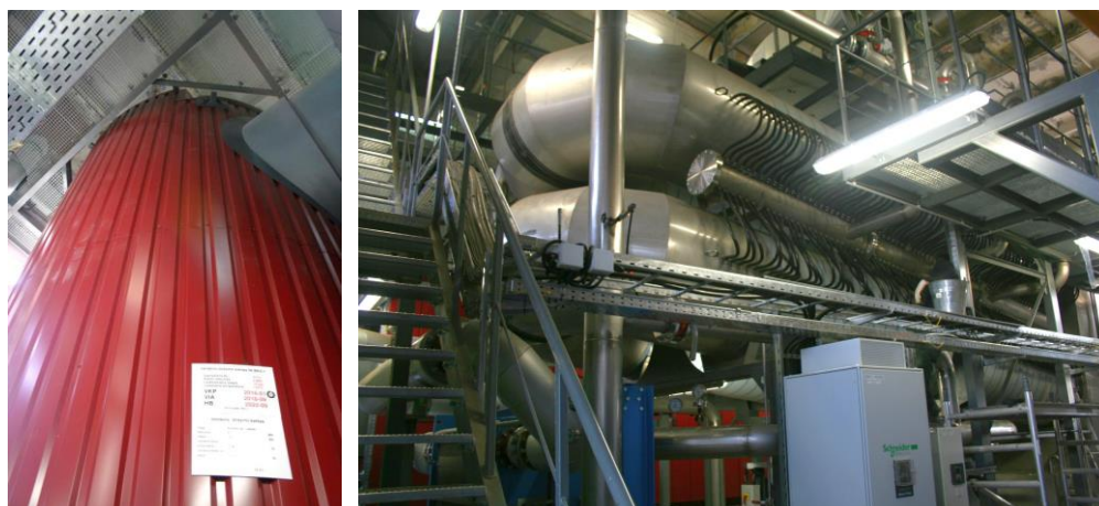
Photo: new water heating boiler and condensational economizer in Šilkas boiler-house
