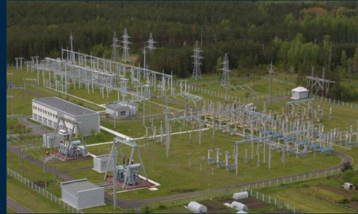
TS – transformer substation
