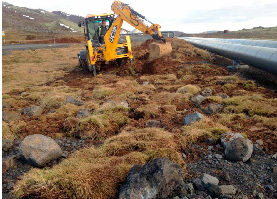
Clumps of vegetation from Hverahlíð utilised for finishing drilling platforms in Hellisheidi
