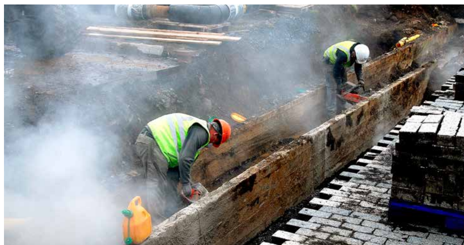
Figure 10. Work at the hot water duct in Rofabaer, Reykjavik. Photo: Hildur Ingvarsdóttir.
