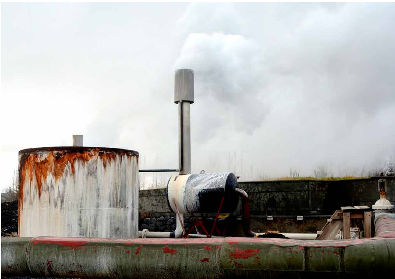
Figure 39. Muffler and steam hood in Hveragerdi. Photo: Bjarni Línal.
