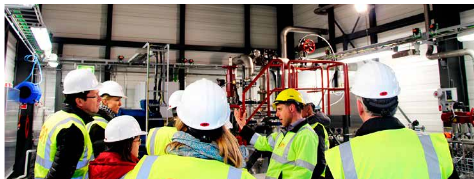
Figure 8. From the opening of the hydrogen sulphide abatement unit at Hellisheidi Geothermal Power Plant. Photo: Thorvaldur Árnason.
