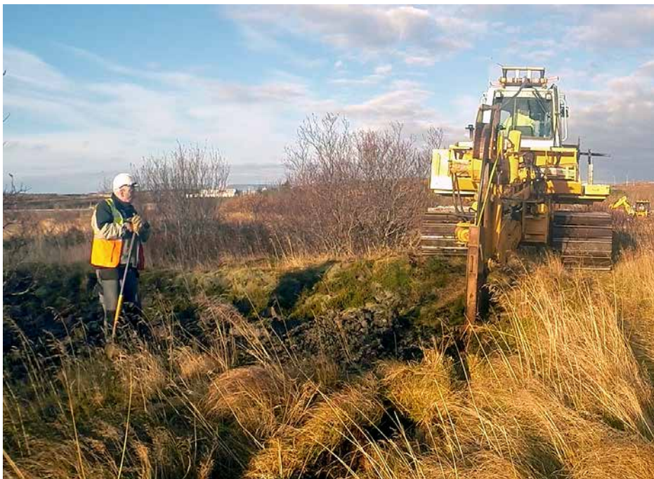
Figure 9. The Ellidavtn Power Line laid underground in the autumn 2014. Technology and work procedures were carefully utilised to minimise the disturbance on vegetated land. Photo: Ingvar Jón Ingvarsson.
