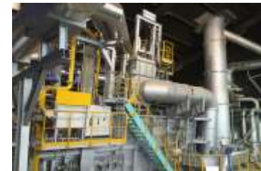
Clervaux remelter investment - improved recycling capabilities
