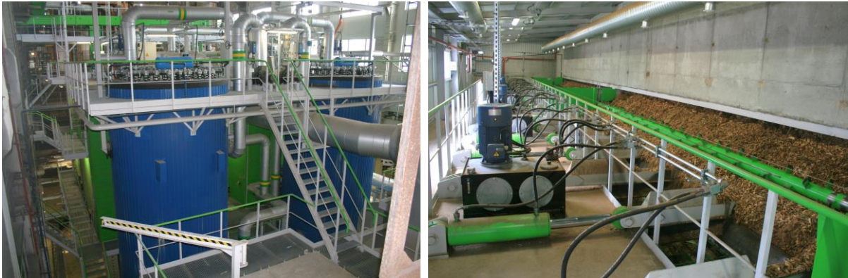
Photo: new water heating boilers and biofuel taking equipment in Petrašiūnai power-plant
