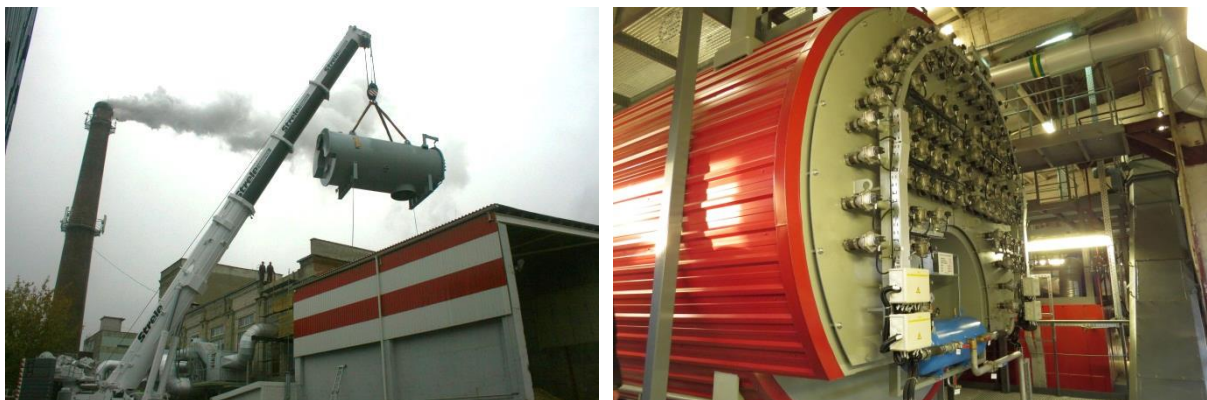
Photo: new biofuel burned water heating boiler is being lifted through the roof of boiler-house and already assembled in its' place
