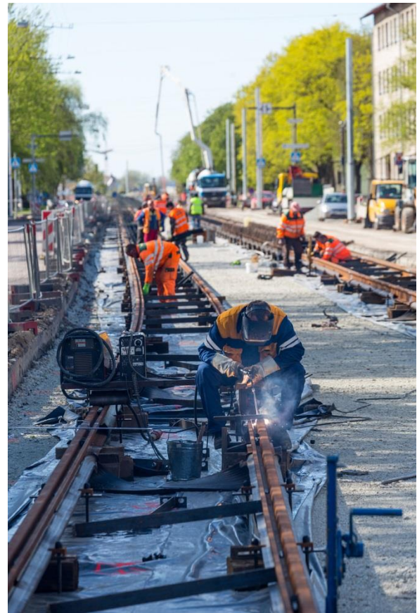
DESIGN AND RENOVATION WORKS OF THE INFRASTRUCTURE OF TALLINN TRAM LINE NO. 4 COMPLETED IN 2015.
