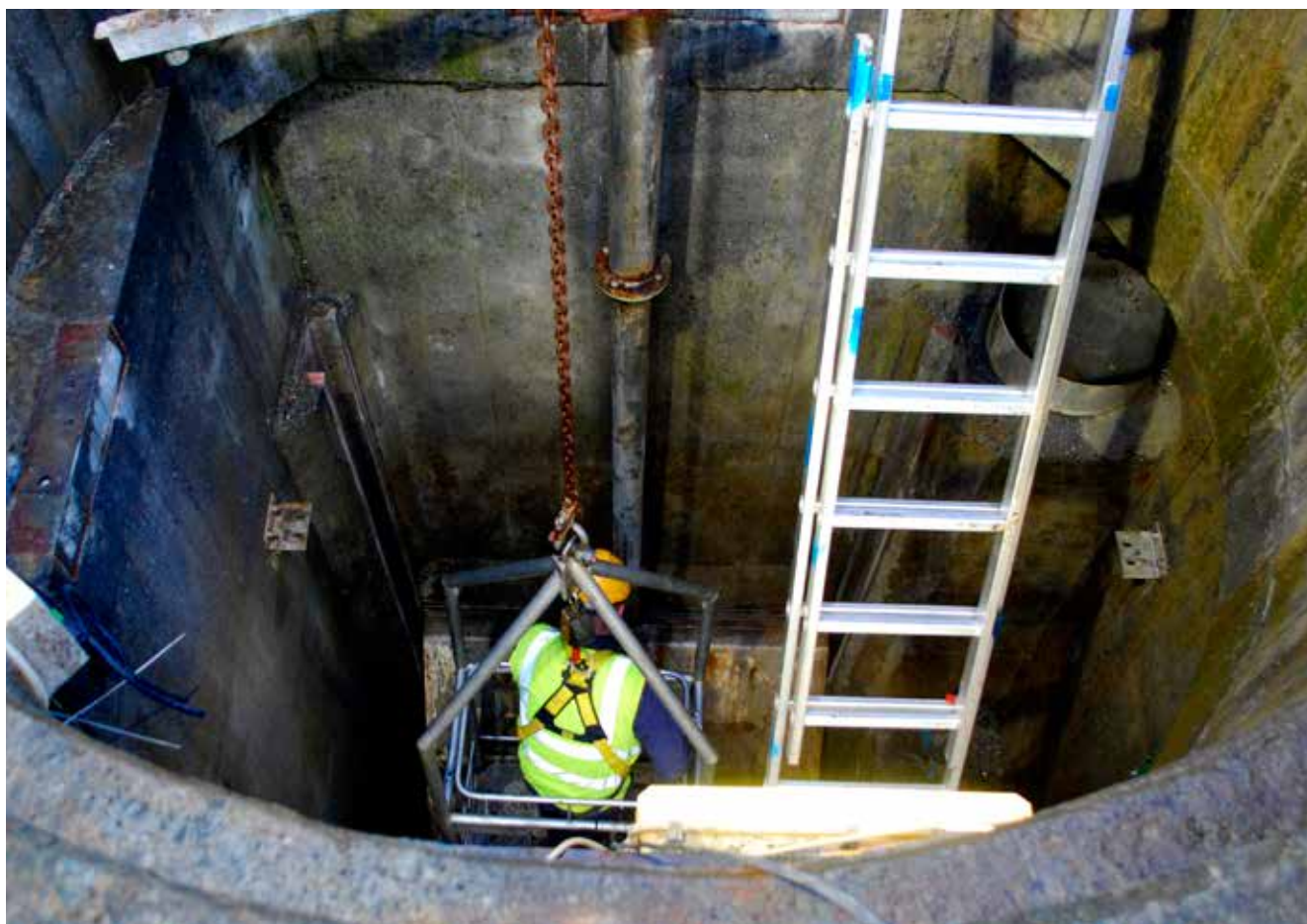
Figure 14. Changing emergency outlet valve of the pumping station in Ingólfsstraeti in Reykjavik. Photograph: Hildur Ingvarsdóttir.
