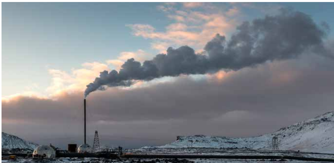
Figure 22. Steam hood ejector near Hellisheidi Geothermal Power Plant. Photograph: Gretar Ívarsson.
