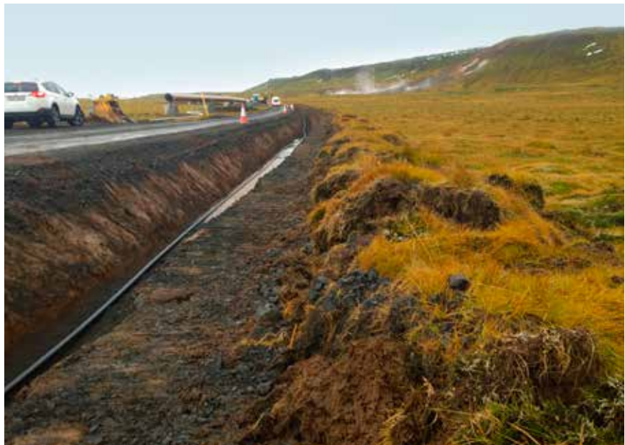
Figure 5a. During construction, strips of turf were removed from the ditch by Hverahlíð and placed on the edge of the ditch. Photograph: Magnea Magnúsdóttir.
