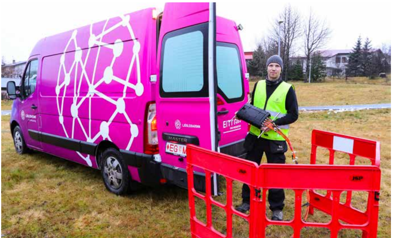
A technician from the Reykjavik Fibre Network performing maintenance work on a cable pit in Seljahverfi in Reykjavik. Photograph: Valur Heidar Sævarsson.
