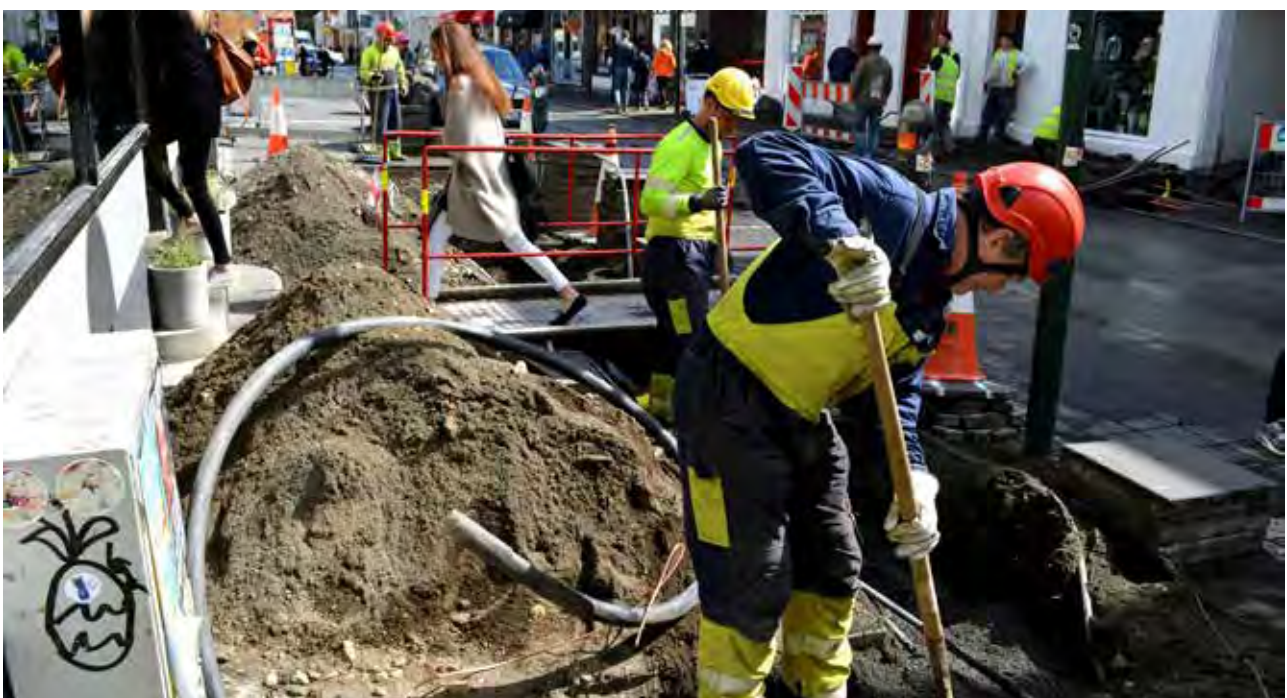
Working on the renovation of the electricity grid in the centre of Reykjavik. Photograph: Hildur Ingvarsdóttir.
