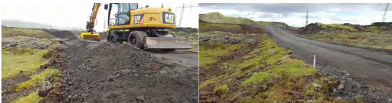
Figure 3. During construction, strips of turf were removed from a road path by Hellisheidi and placed on the edge of the road after construction. Photograph: Magnea Magnúsdóttir.
