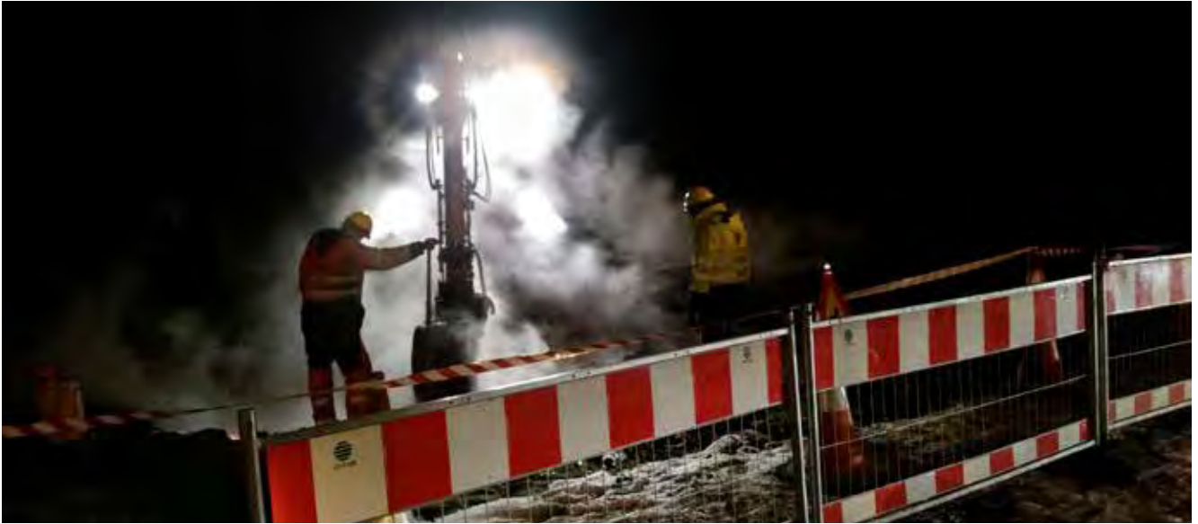
Working on a hot water utility in Reykjavík. Photograph: Bjarni Líndal Snorrason.
